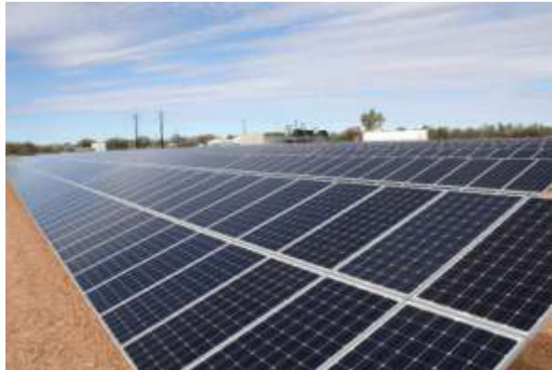
Fig. 1 - Ti Tree Solar Power Station. GSS and diesel power station in background.
